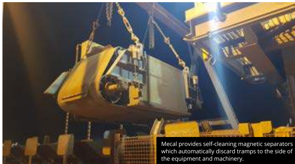
A magnetic separator above a conveyor belt removing tramp metal from material.
