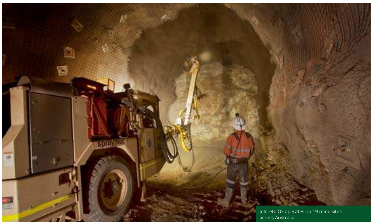
Jetcrete Oz has been the shotcrete contractor of choice for Australian miners for more than three decades.
