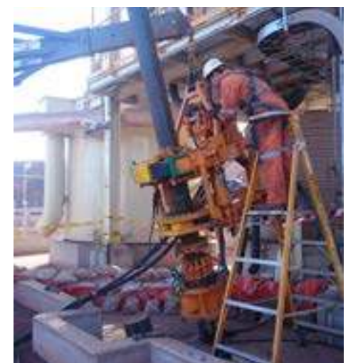
AGE Developments provides a complete design, manufacturing, installation, and retrieval turnkey service for paste fill bores with an extensive track history.
