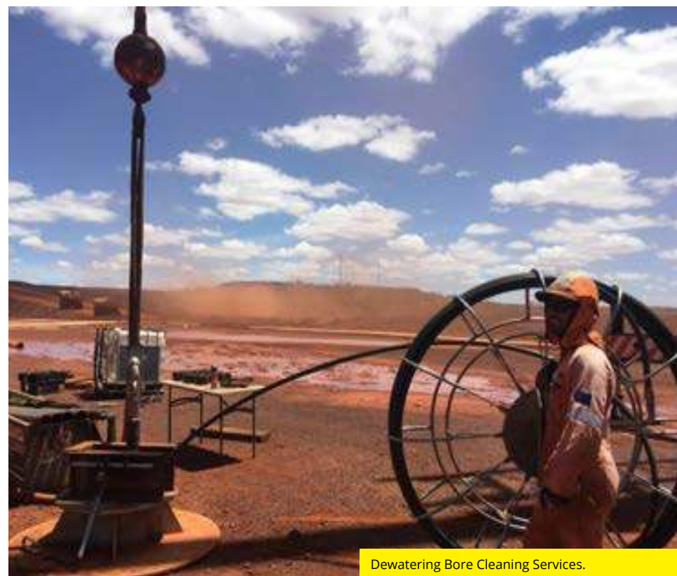
ESP, cable and Wellmaster pump column fishing with aid of specialist tooling and real-time downhole CCTV camera system.
